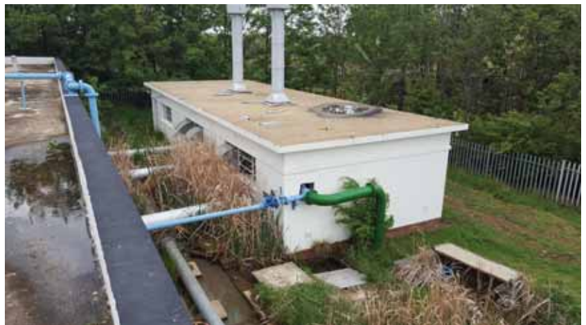
Clear water pump house
