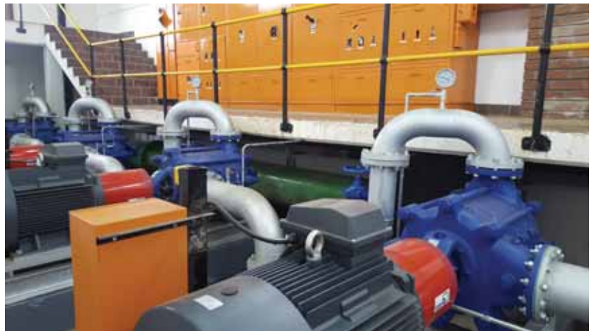
Upgraded Clearwater pumps
