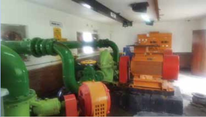
Clearwater pumps requiring upgrade
